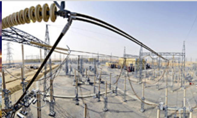
Grid sector Equipment & services for power transmission
